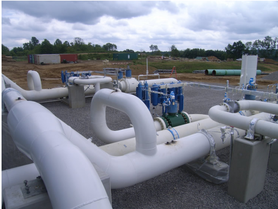
Figure 2 Regulation and Measurement Station
