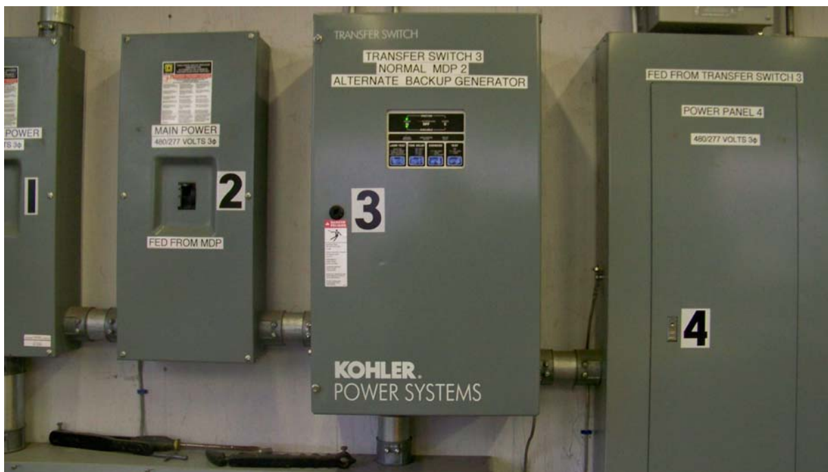
Liberty Keene – The system was not configured to transition to emergency backup power without experiencing a brief power interruption to the variable speed drives which requires manual restart of the blowers.
