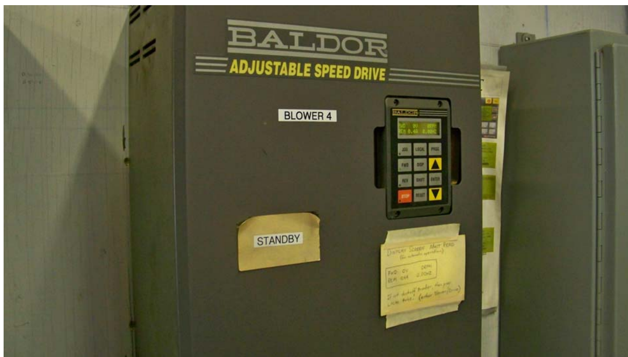
Liberty Keene - The blowers are equipped with variable speed drive controls that are sensitive to incoming 3-phase power fluctuations.
