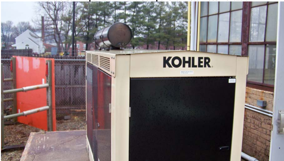
Liberty Keene – The air blowers are equipped with a 125 KW emergency generator.
