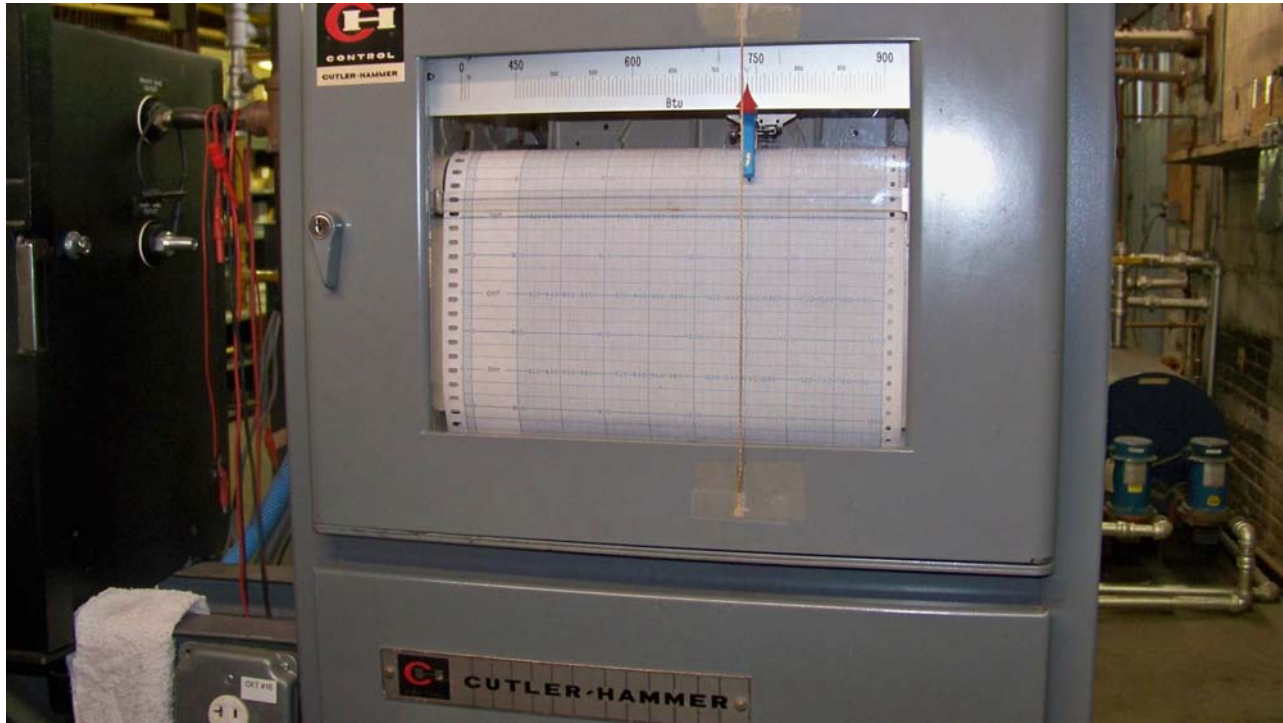
Liberty Keene – The plant propane/air output Btu heating value is monitored and recorded using a Cutler-Hammer calorimeter.
