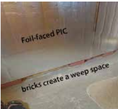
PIC foundation insulation: Installers glue PIC-foam sheets to the concrete wall, and they leave a weep space at floor level.
