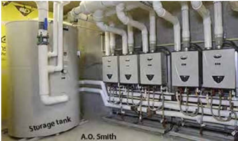
Popular multifamily water-heating solution: On-demand water heaters heat water for a storage tank and for demand in a medium-sized multifamily building.
