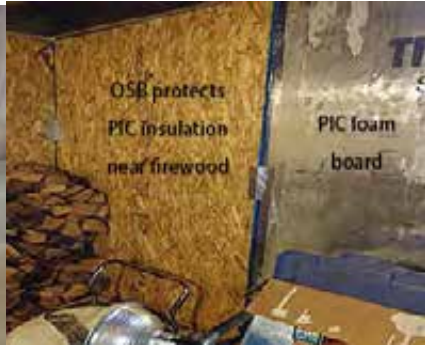
Protecting PIC foam: Installers attach OSB to protect PIC-foam sheets from firewood storage.
