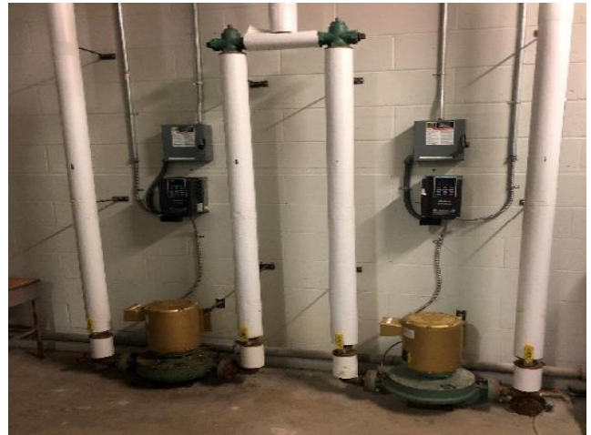
Above: Before (left) motor starters and after (right) with new variable frequency drives
