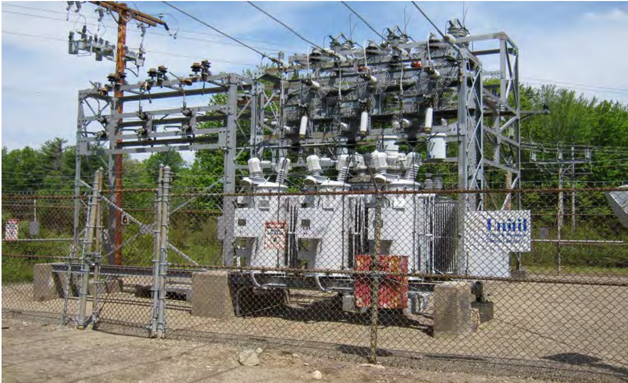
Figure IV-6 – 34.5kV to 13.8kV Unilt electric distribution substation located in East Kingston, New Hampshire. (Photo by NEI-Unilt System)
