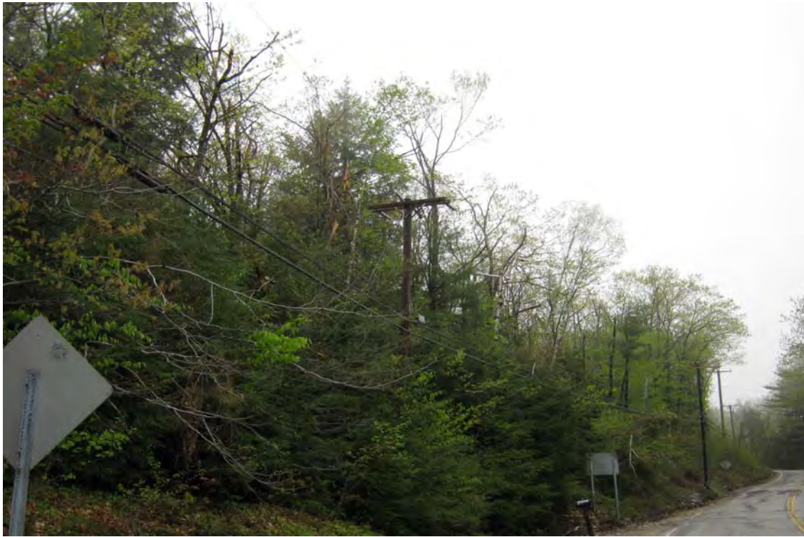
Figure IV-5 - Typical PSNH distribution circuit near Greenville, New Hampshire. (Photo by NEI - PSNH System)
