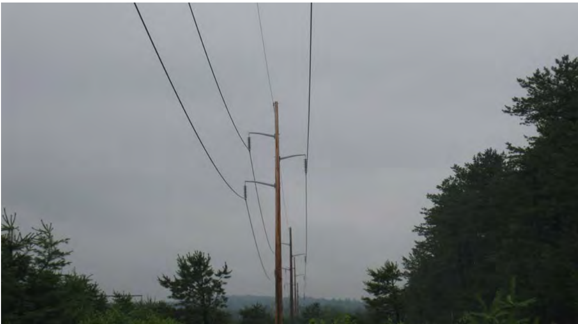
Figure V-10 - PSNH 115kV circuit V182 in Concord, New Hampshire. (Photo by NEI)
