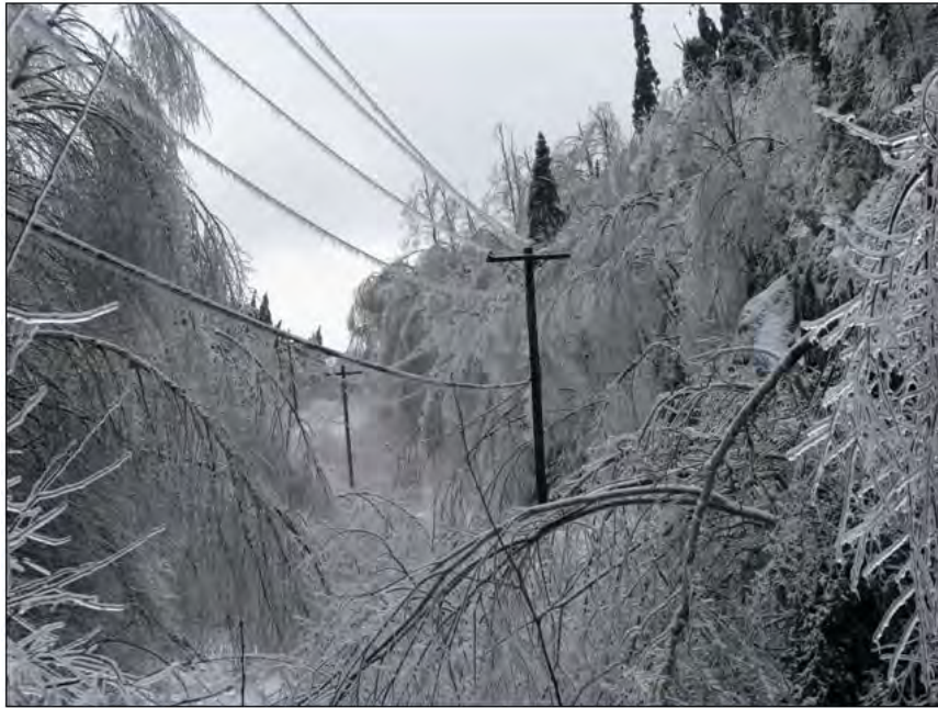
Figure I-2 – Damage in PSNH distribution line corridor. (Photo courtesy of PSNH. Exact location unknown.)
