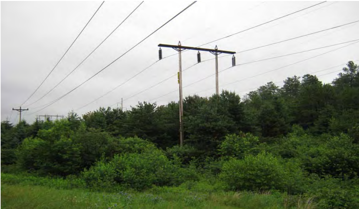
Figure V-11 - Northeast view of PSNH 115kV circuit P145 with circuit V182 shown in the background. (Photo by NEI)
