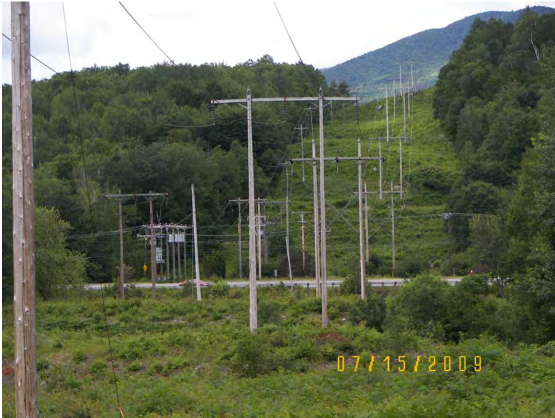
Figure IV-2 - Common H-Frame transmission line construction. (Photo courtesy of NHPUC)
