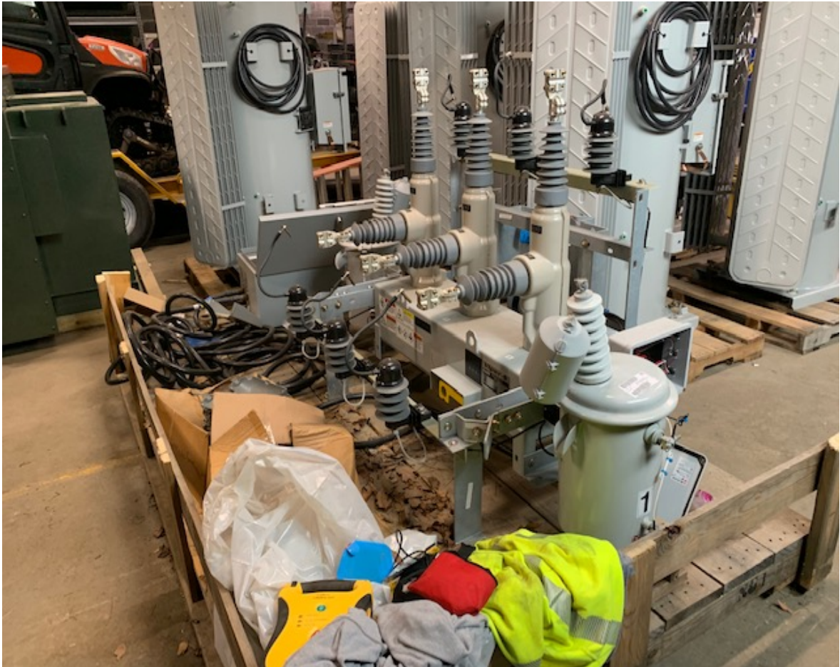
Photo 4 courtesy of PUC Safety Division taken 3/6/2020. Photo inside of the warehouse at the Lebanon Area Work Center. The photo shows the electrical equipment assembly consisting of Viper S interrupters, lightning arresters, potential transforms, control and electrical feed cables, and electronic control box. Photo 4 taken from the opposite location of Photo 1
